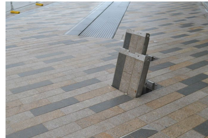
■ In-ground power unit
