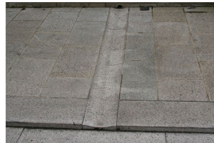
--- Dished granite surface gully
