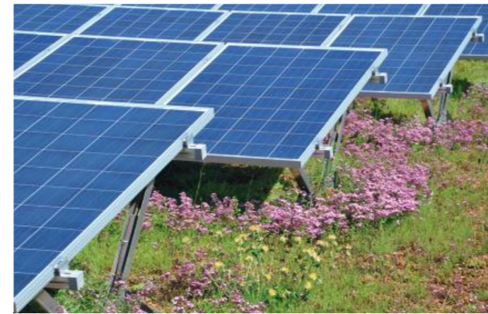
PV panels on green roof mat
